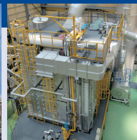
VOLCANO Combustion Test Site responsible for verification testing during the development of MECS-GCU
